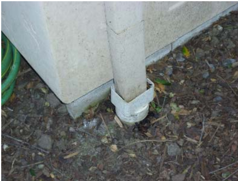
Sub-surface drain system
