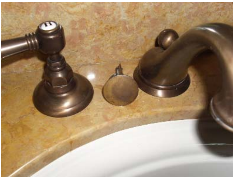
Drain stop needs repair
