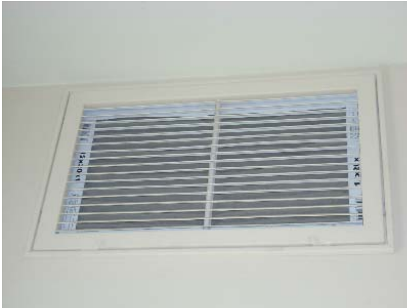
Air filter replacement recommended
