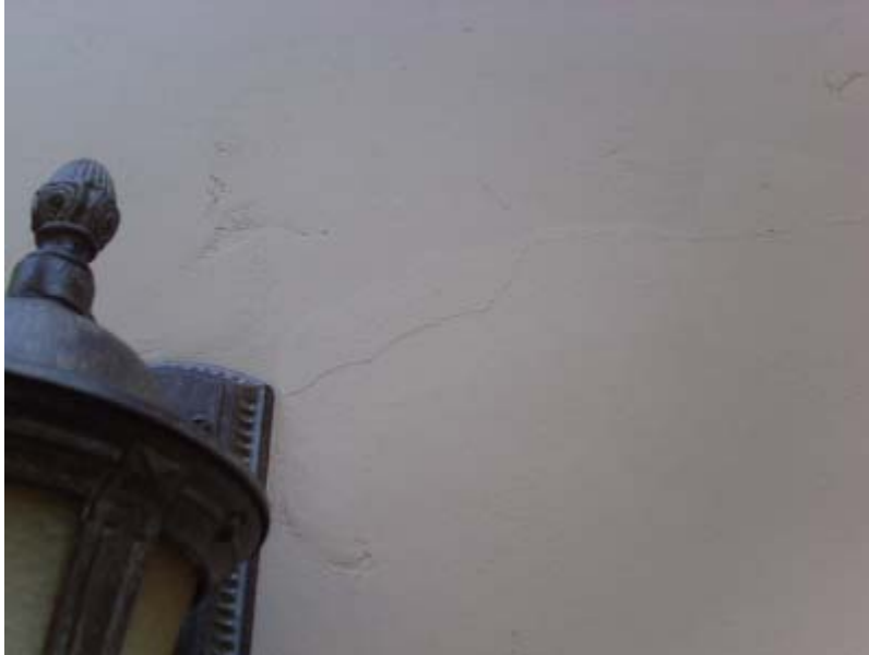
Small stucco cracks noted
