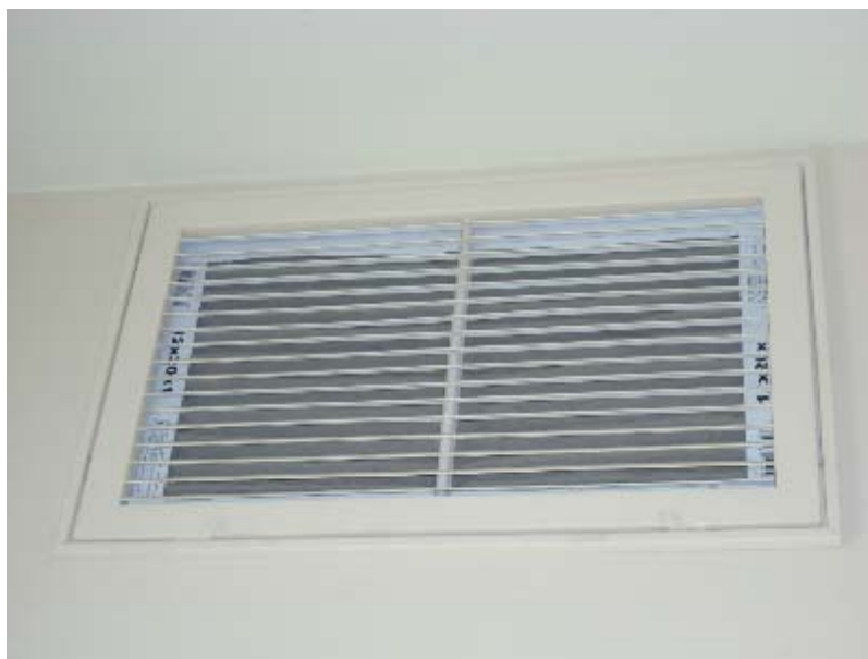
Air filter replacement recommended
